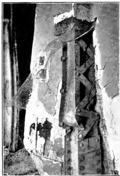
AN INSUFFICIENTLY PROTECTED STEEL COLUMN AFTER A FIRE.
